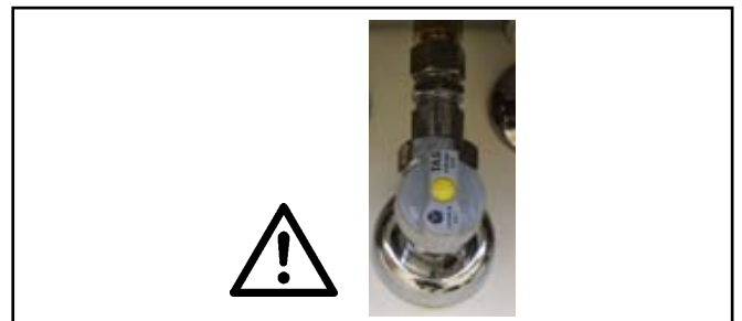
Figure: Gas connection
